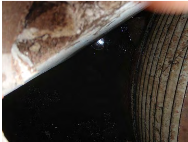
Photo 4: Underground Void at BH13.
